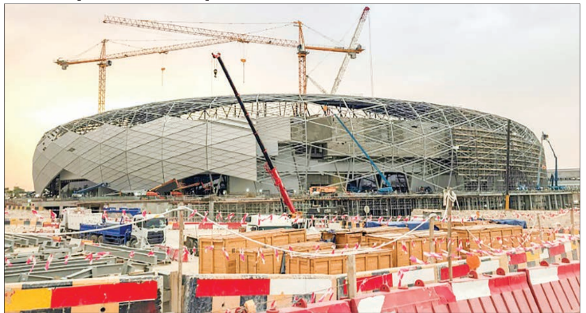
The Education City stadium, seen here under construction in May last year, is the third to be completed among eight venues Qatar is readying for the 2022 World Cup. PHOTO: AFP
