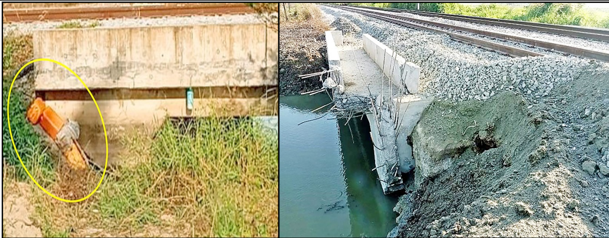
Damages of the railway track between Daik-U and Pyuntasa Stations in the remote mine attacks of the terrorists
