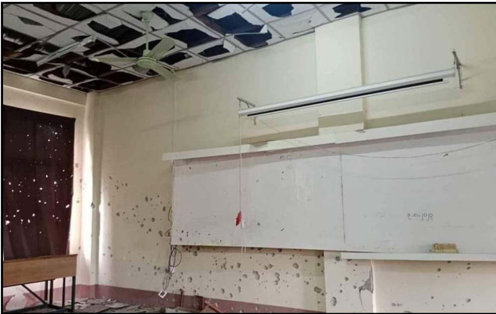
The image that KNPP and PDF terrorists raided non-military target of Loikaw University resulting educational buildings damaged, posted on the social media as the evidence
